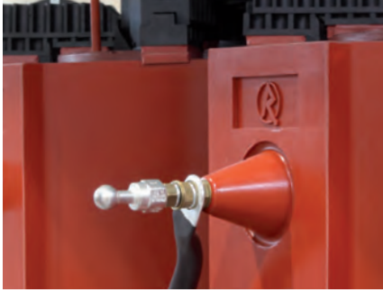
HV winding connections with ball connection bolts
